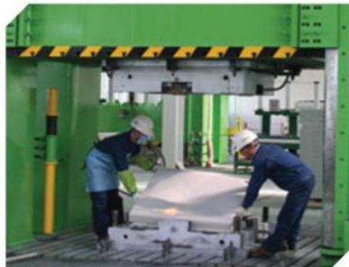
Ejecting Molded Panel After certain time of molding, take out the molded panel from molds.
